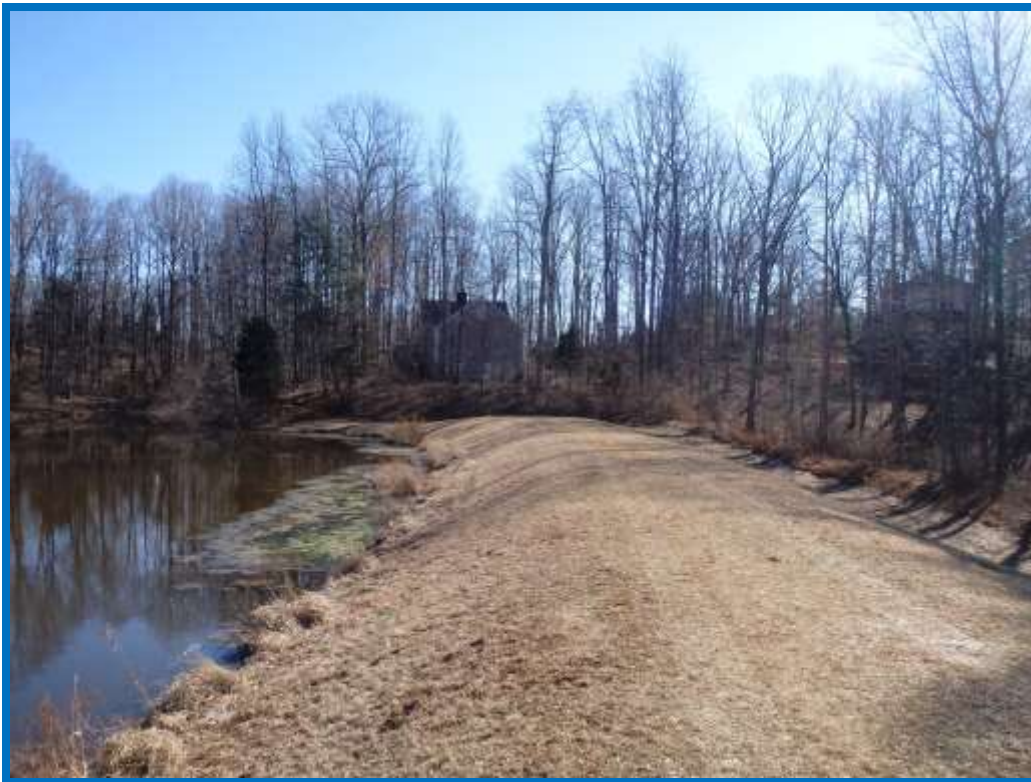
Figure 30 - Looking across the crest of the dam towards left abutment and auxiliary spillway
