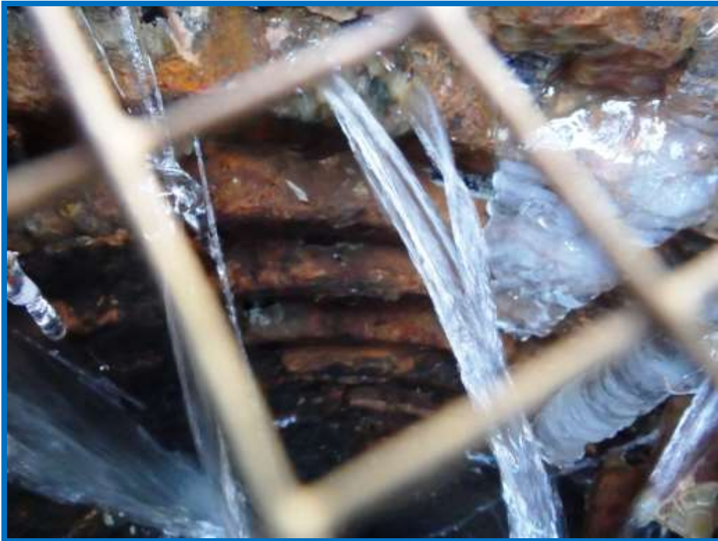
Figure 4 - Picture of small pinhole leaks near top of riser
