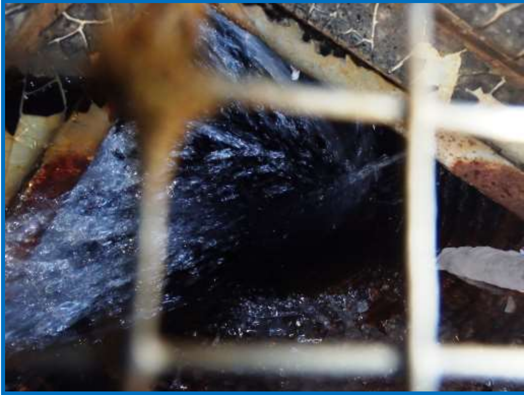
Figure 3 - Looking down into riser before water was controlled
