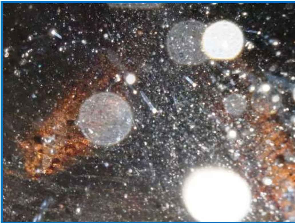
Figure 8 - Close-up of seeps in riser, approximately half-way down pipe
