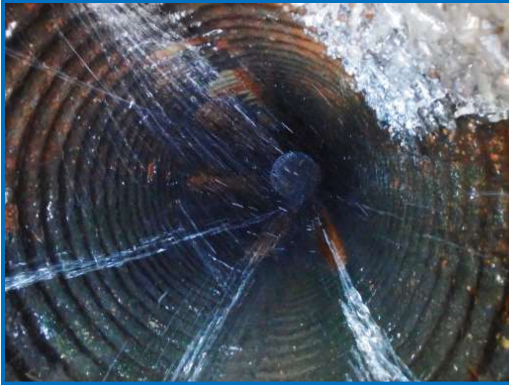
Figure 7 - Looking down into riser, note small seeps as evidence by brownish color
