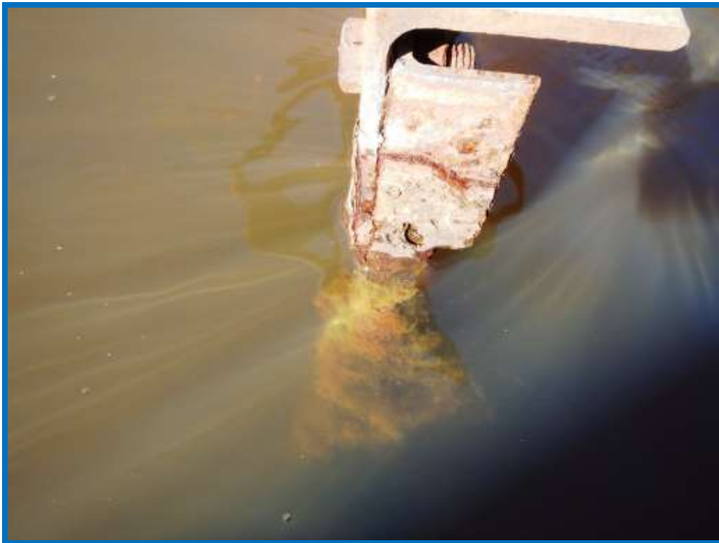
Figure 12 - Sluice Gate Frame is deteriorated
