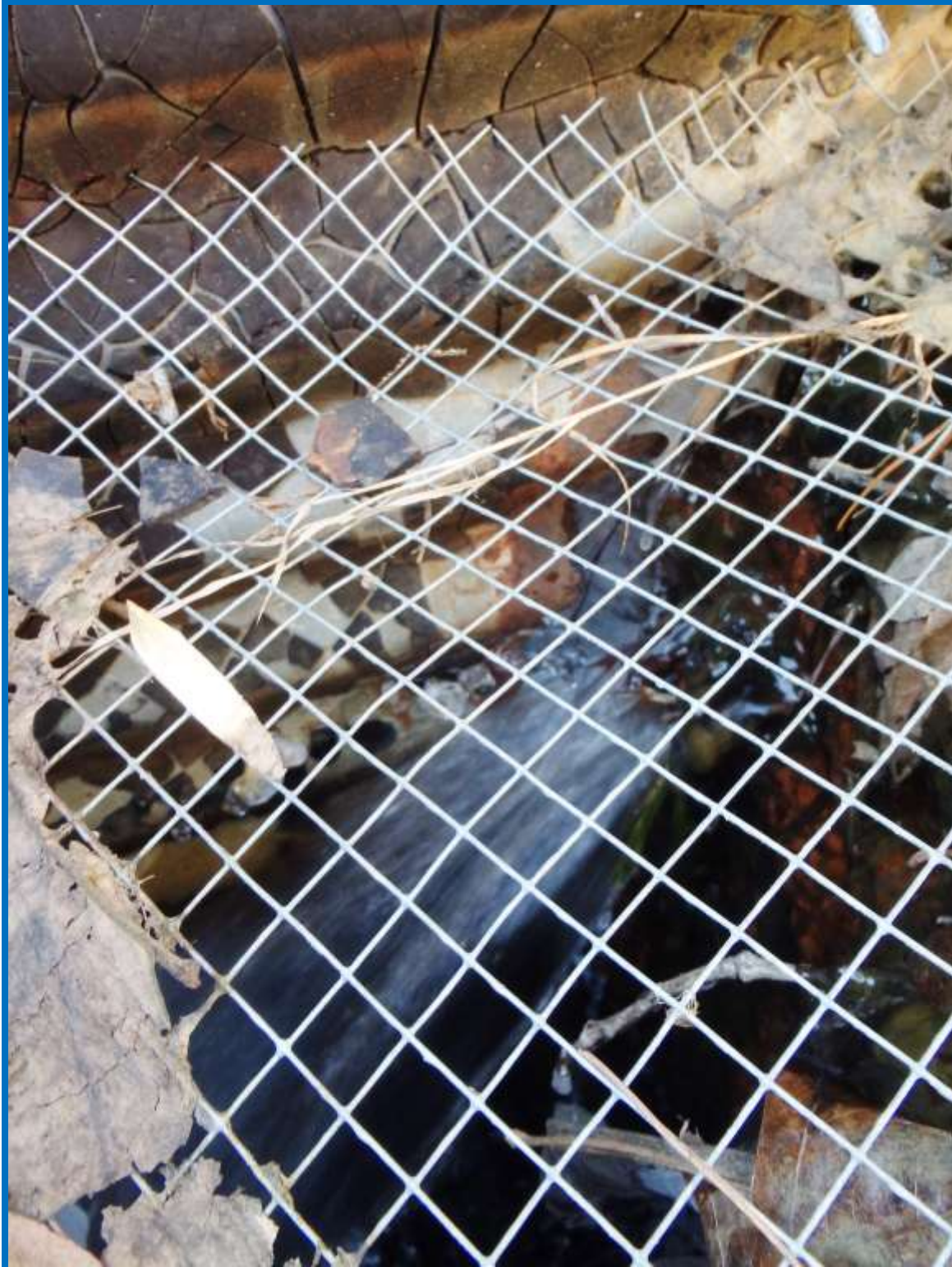
Figure 5 - Larger leak in riser
