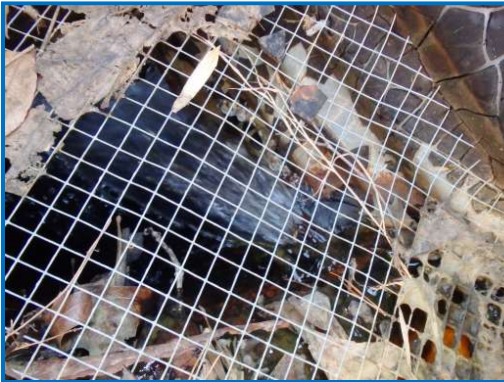
Figure 2 - Screen installed on top of trash rack
