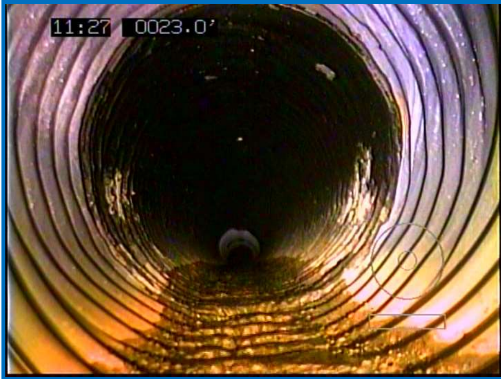
Figure 19 - Picture at Transition from new to old CMP
